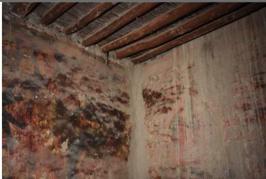
Fig 6. Dust and dirt depositoin on the painted surface due to leaking roof.
