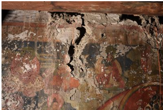
Fig 4. Detachment and flaking of paint layer. North wall of the shrine, first floor.
