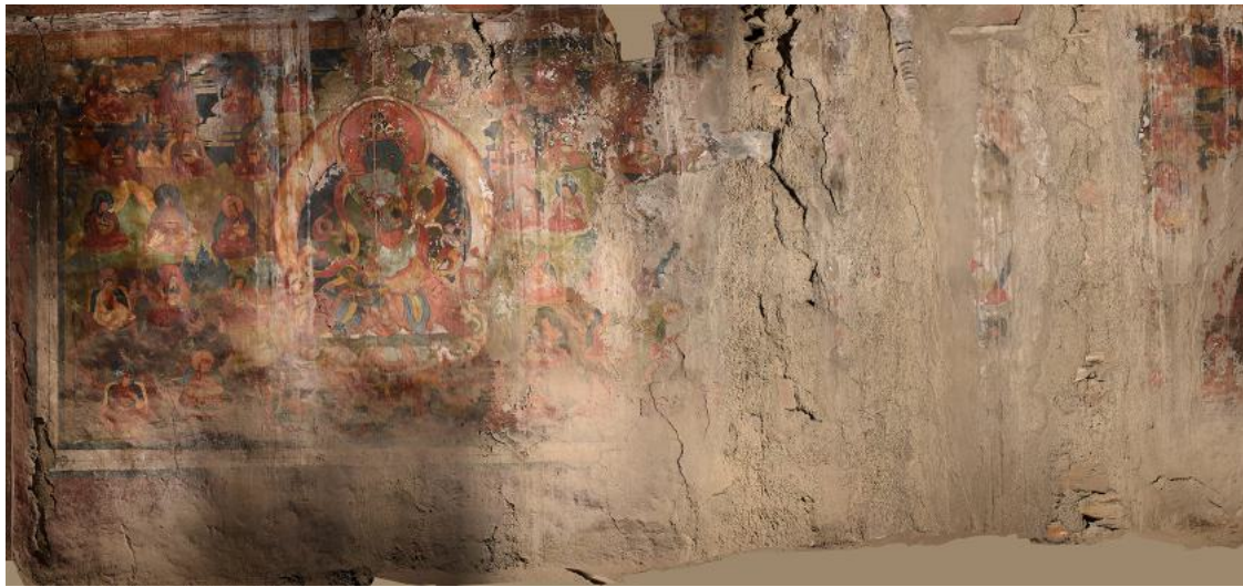
Fig 3. Highly damaged paintings in the first floor of the shrine, north wall. Images merged by photogrammetry.
