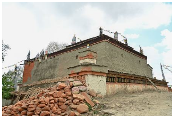
Figure 24: The temple after the repair of all mani wheels and chörten as well as plastering the temple.
