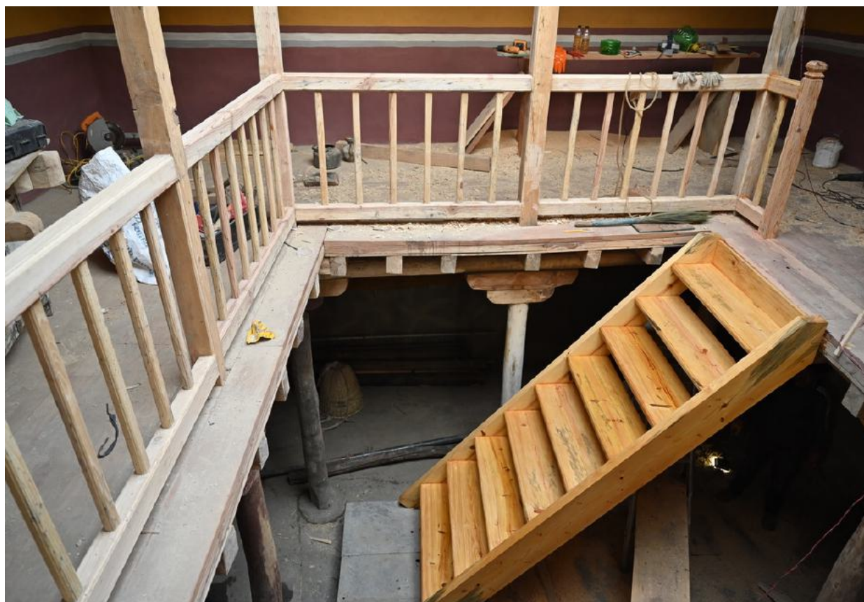
Figure 20: View of the new railing and staircase in the atrium of the caretaker's area.
