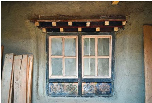
Figure 10: The window in the guest lobby before repainting.
