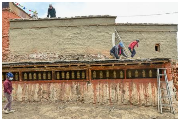
Figure 23: Repair of the mani wheels to the back of the caretaker's quarter.
