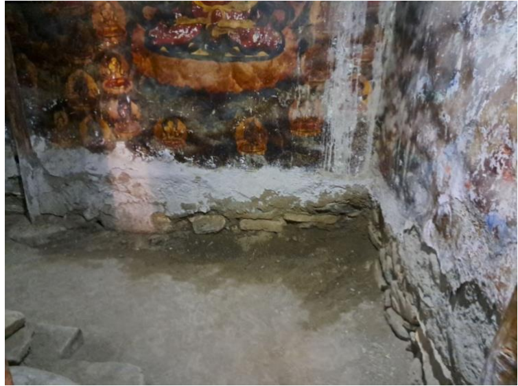
Figure 4: Water entered the building behind the main Buddha image as seen on October 15.
