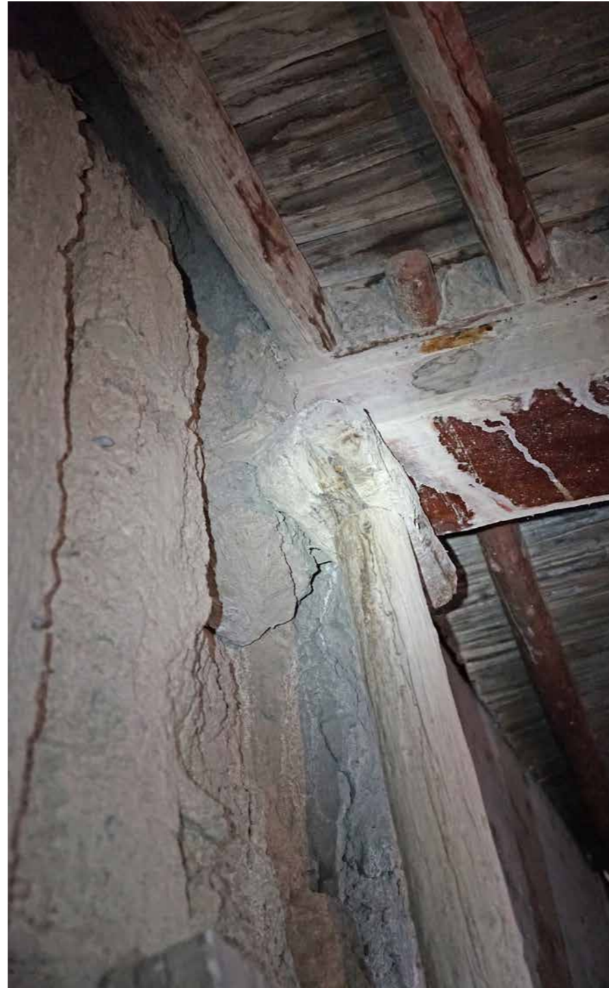
DETAIL OF THE NORTH WALL AND BEAM The wall has been eroded to a point that is can't provide sufficient bearing for the cross beam. The beam is currently held up by a temporary prop.
