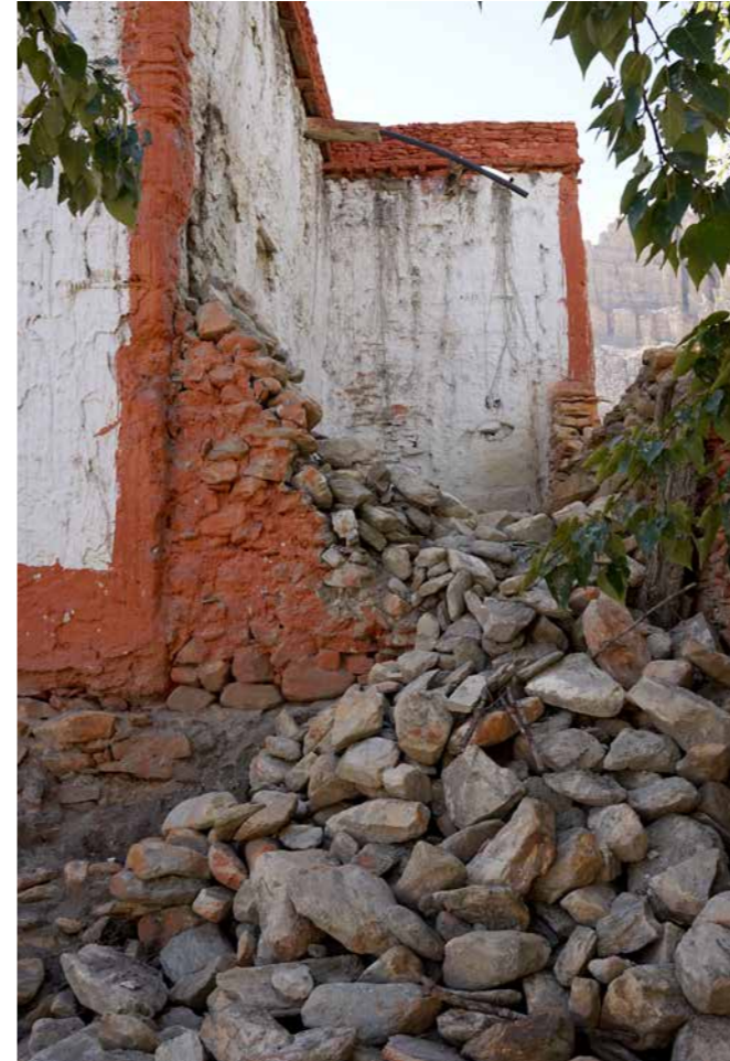
NORTH-EAST CORNER The partly collapsed stone wall enclosure will be completely removed which will allow better drainage from the roof water spouts.
