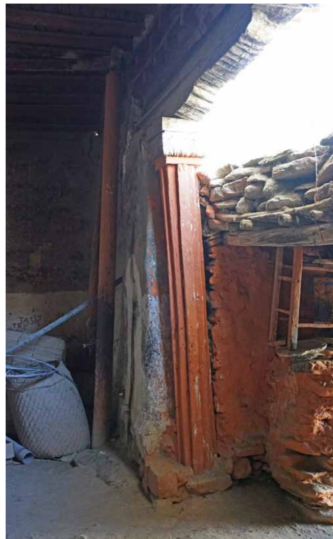
CROSS BEAM AND TEMPORARY SUPPORTS The badly damaged column is not original to the buildings. It leans to the left whereas the capital has tilted in the opposite direction. The base stone was obviously only temporarily
