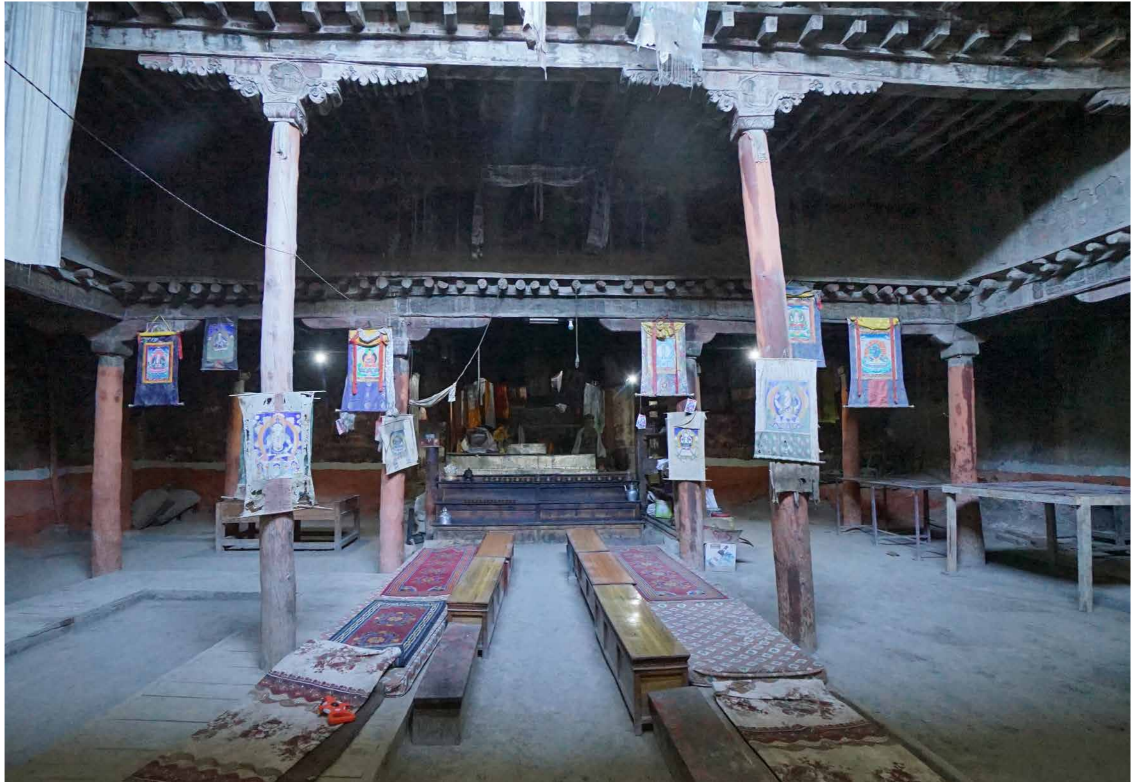
MAIN HALL, VIEW TOWARDS THE WEST Gaps between capitals and beams indicate the settlements of the bearing structure. The columns in front are leaning which likely is a result of earthquake damage. The right cross beam sags which is probably caused by wet rot. Water damage is evident throughout the building.
