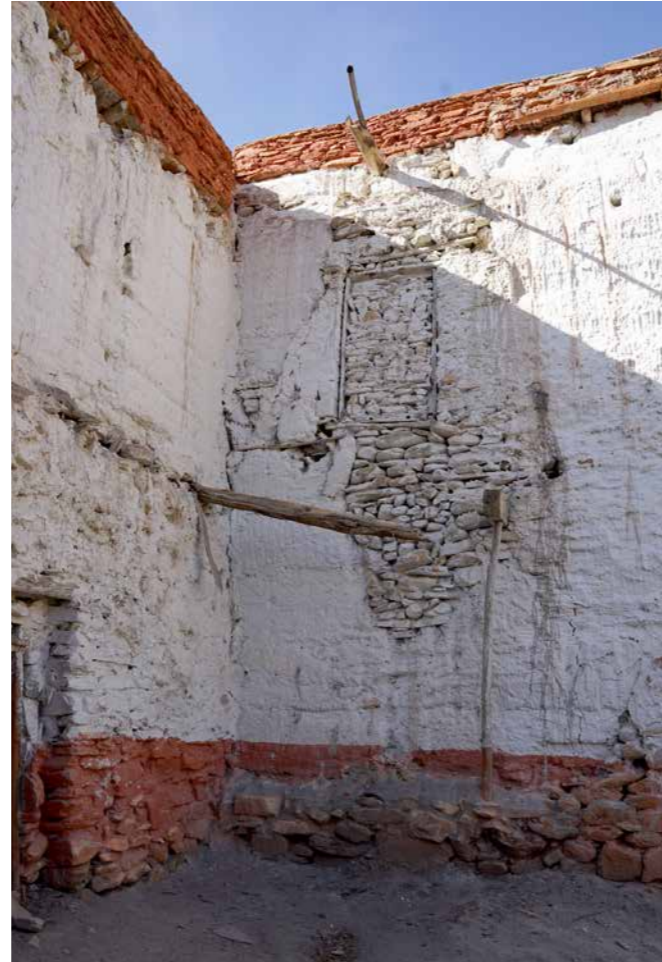
SOUTH-EAST CORNER View from south. The area was once covered by a two-story porch and balcony. Only a single round joist projecting from the wall remains. The wall on the right was heavily eroded by roof leaks. The damaged wall and door formerly leading to the balcony was filled in with stones.
