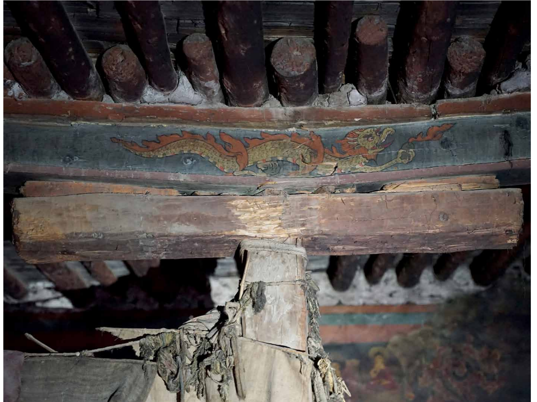
DAMAGE BEYOND REPAIR
