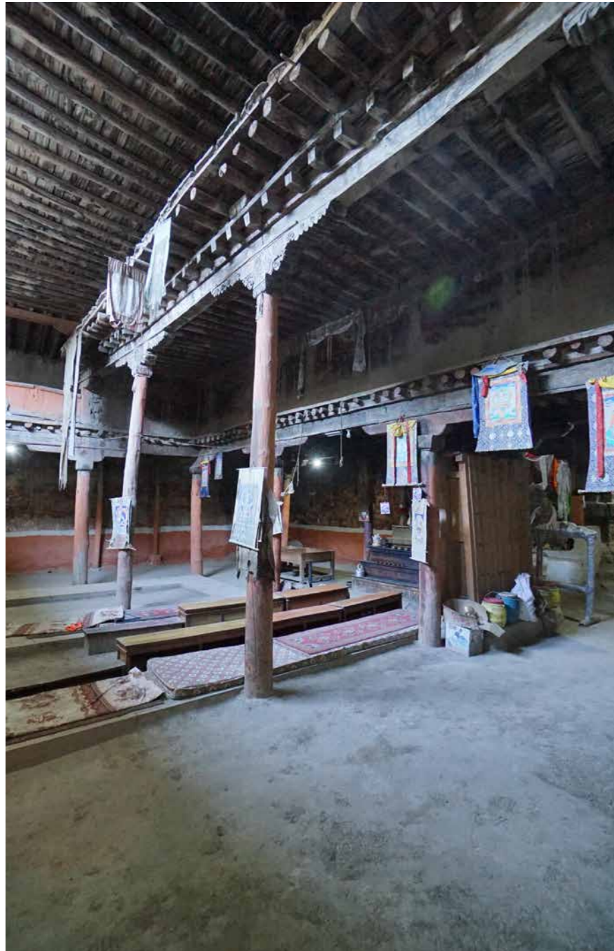
VIEW TO THE SOUTH-WEST The two tall round pillars are leaning. They will be reinstalled on new point foundations.
