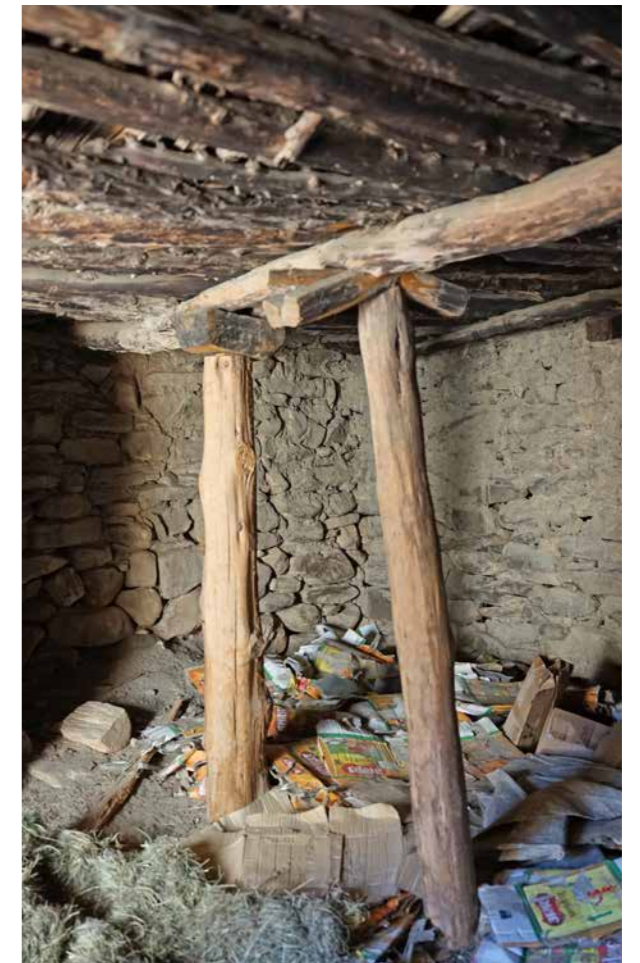
TEMPORARY PROP The temporary supports are affected by wet rot and might give way at any time.
