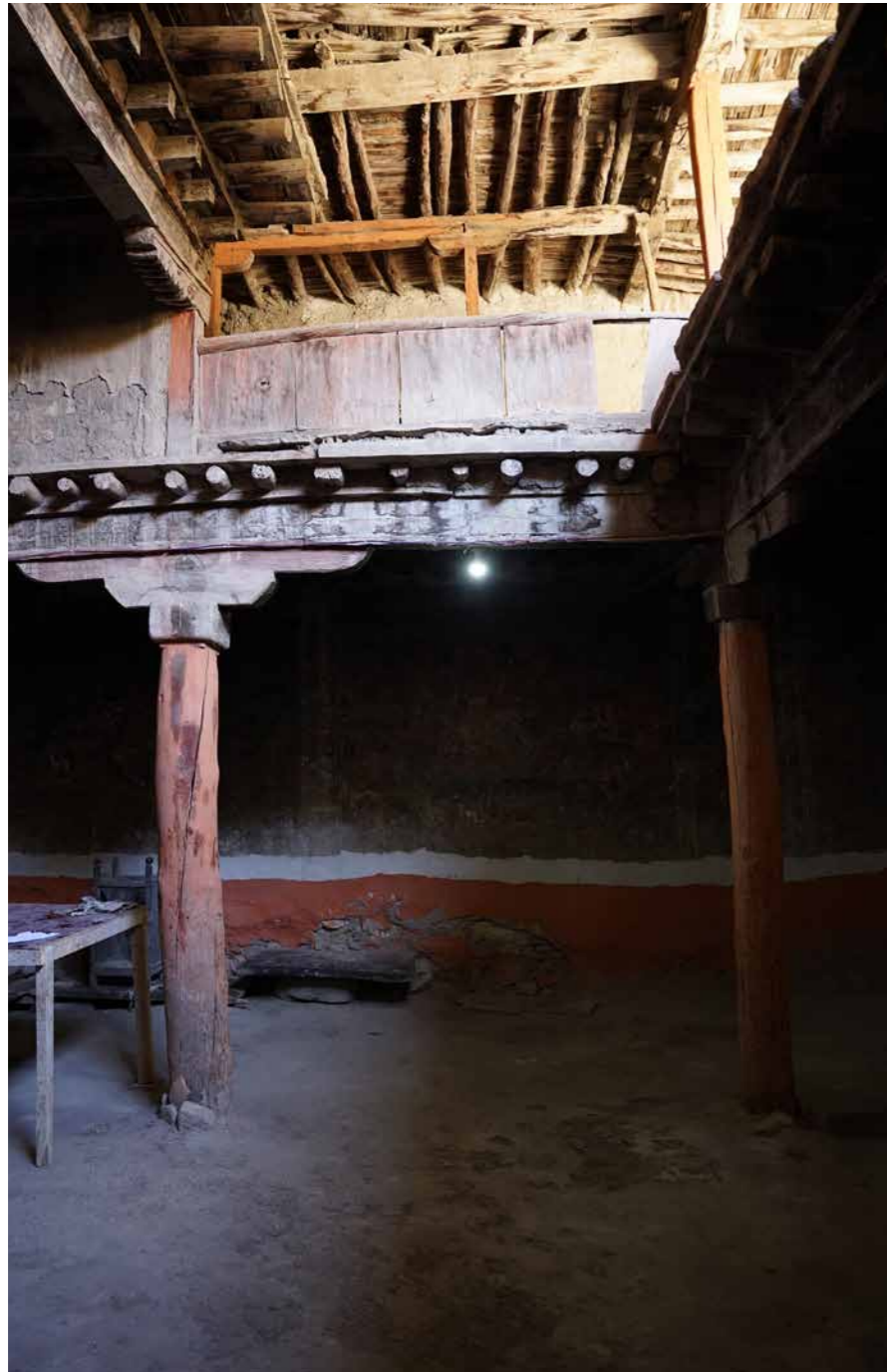
VIEWS OF THE DAMAGED CEILING STRUCTURE The main beam and round poplar joists are held up by temporary supports. Cracks below the beam were poorly patched up with mud mortar.
