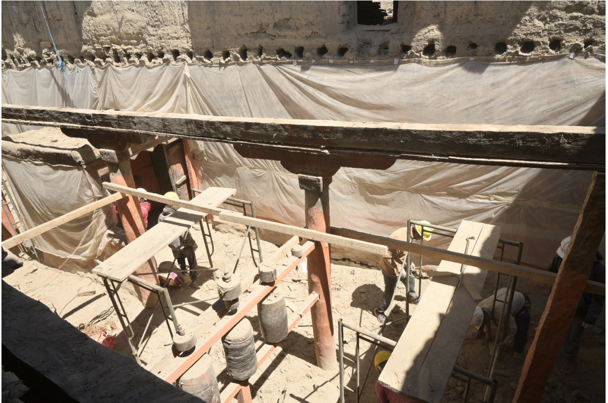
Figure 22: View into the entry area of the Assembly Hall after the dismantling of the two levels above it.
