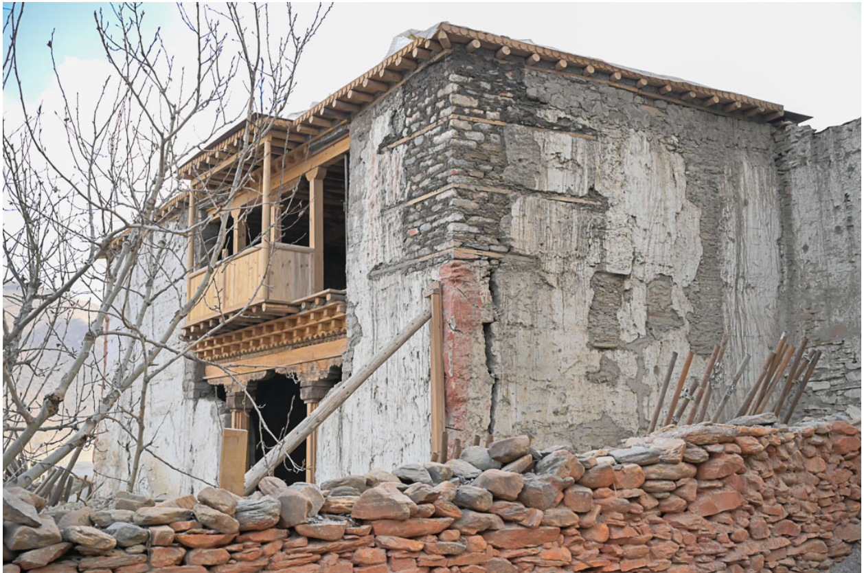
Figure 12: The northeast corner after reconstruction, the crack still visible on the lower floor.
