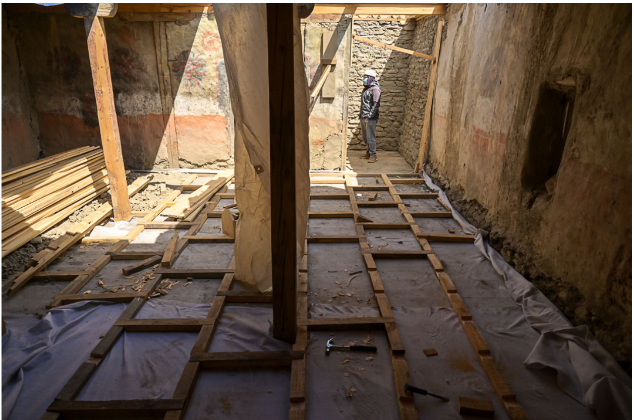
Figure 16: Preparing the wooden floor for the painted room of the south wing.
