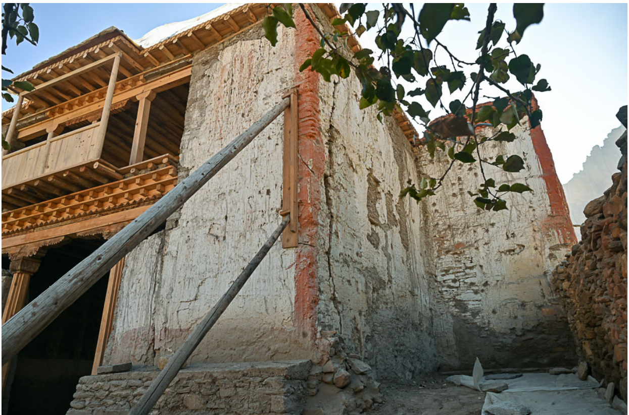
Figure 5: The severe crack at the northeast corner of the Entry Hall in October 2023.
