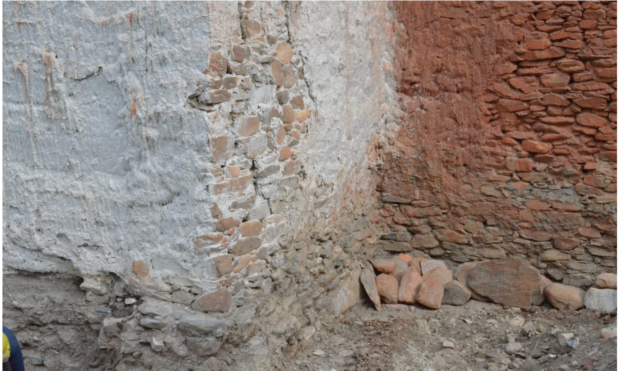
Figure 57: Vie of the northwest corner with the wall cracked and bulging.
