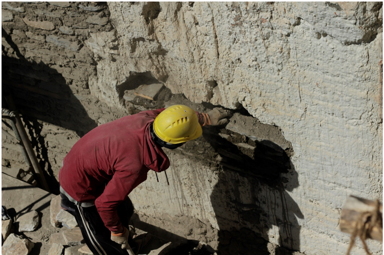
Figure 67: View from top during the repair of a stone wall showing wooden members to connect the repair to the original wall.
