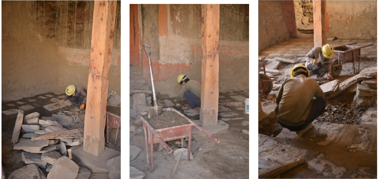
Figure 26: Three images showing the laying of the stone slates on the floor of the Entry Hall.
