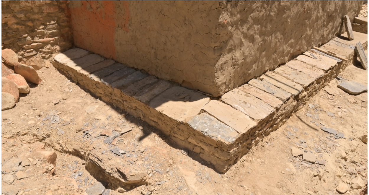
Figure 51: The foundation wall after laying the stone slate upon the mud layer.
