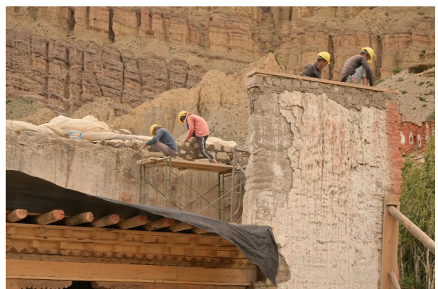
Figure 16: Maintaining the level for the wooden ties on the wall before the top floor joists were placed.
