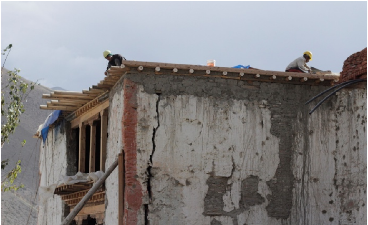
Figure 25: Placing the wooden members with circle design along the top of the wall to support the parapet.
