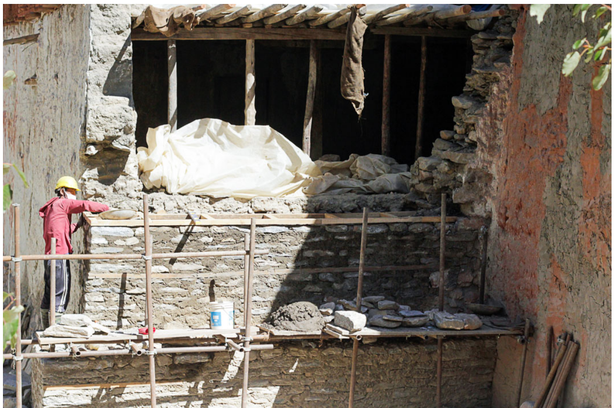
Figure 65: The wall reconstructed to the level of the first floor, where a wall-tie was inserted.
