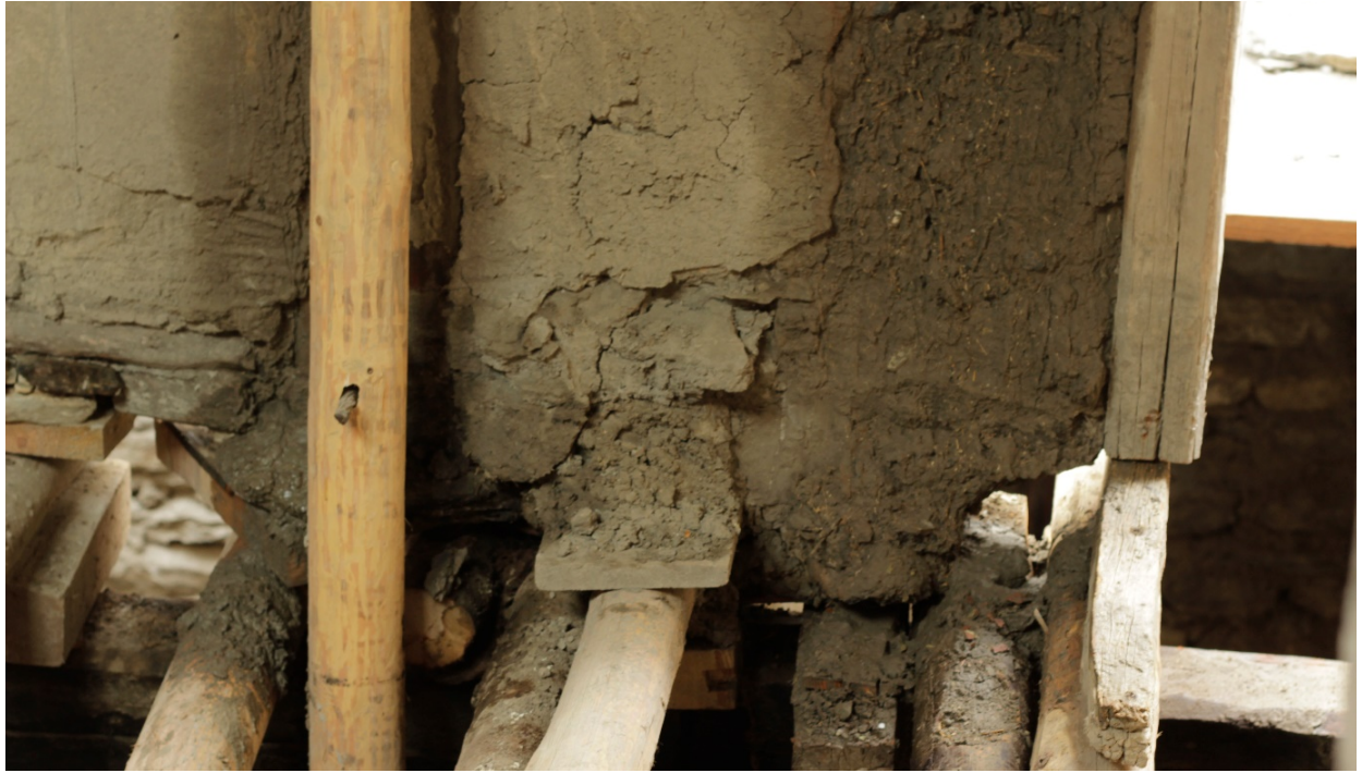
Figure 68: Rain damage to an exposed section of a wall which was repaired later on.
