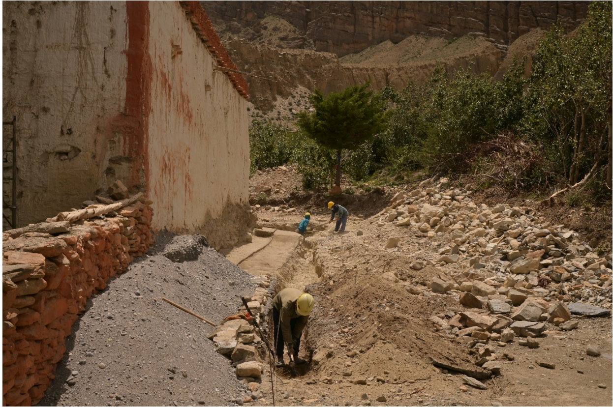
Figure 56: Digging the drainage and foundation for mani-wall on the north side of the monument.
