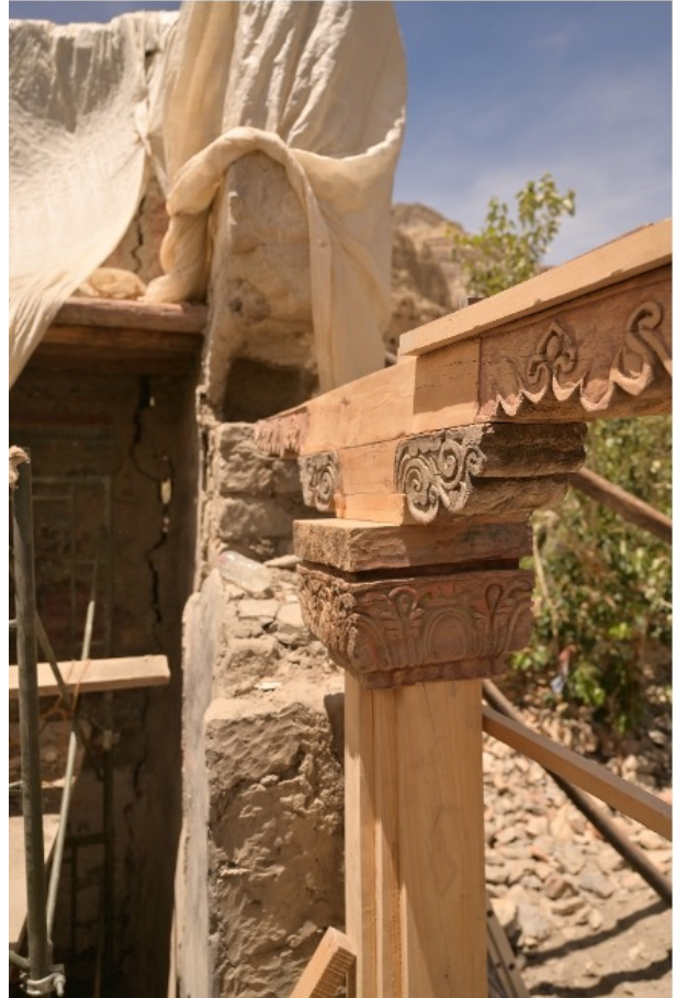
Figure 8: The old capital members placed on the new column aligned with the wall.
