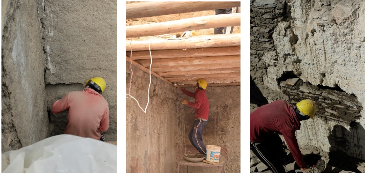
Figure 66: These images show repair work in different areas of the temple using different techniques as required.
