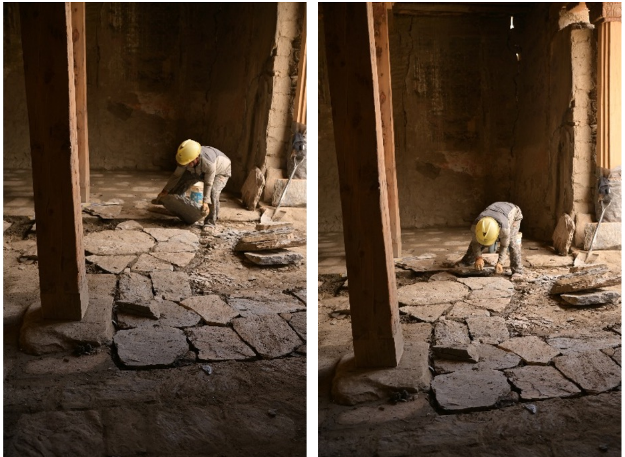
Figure 27: Laying the stone slate floor in the entrance area of the Entry Hall.
