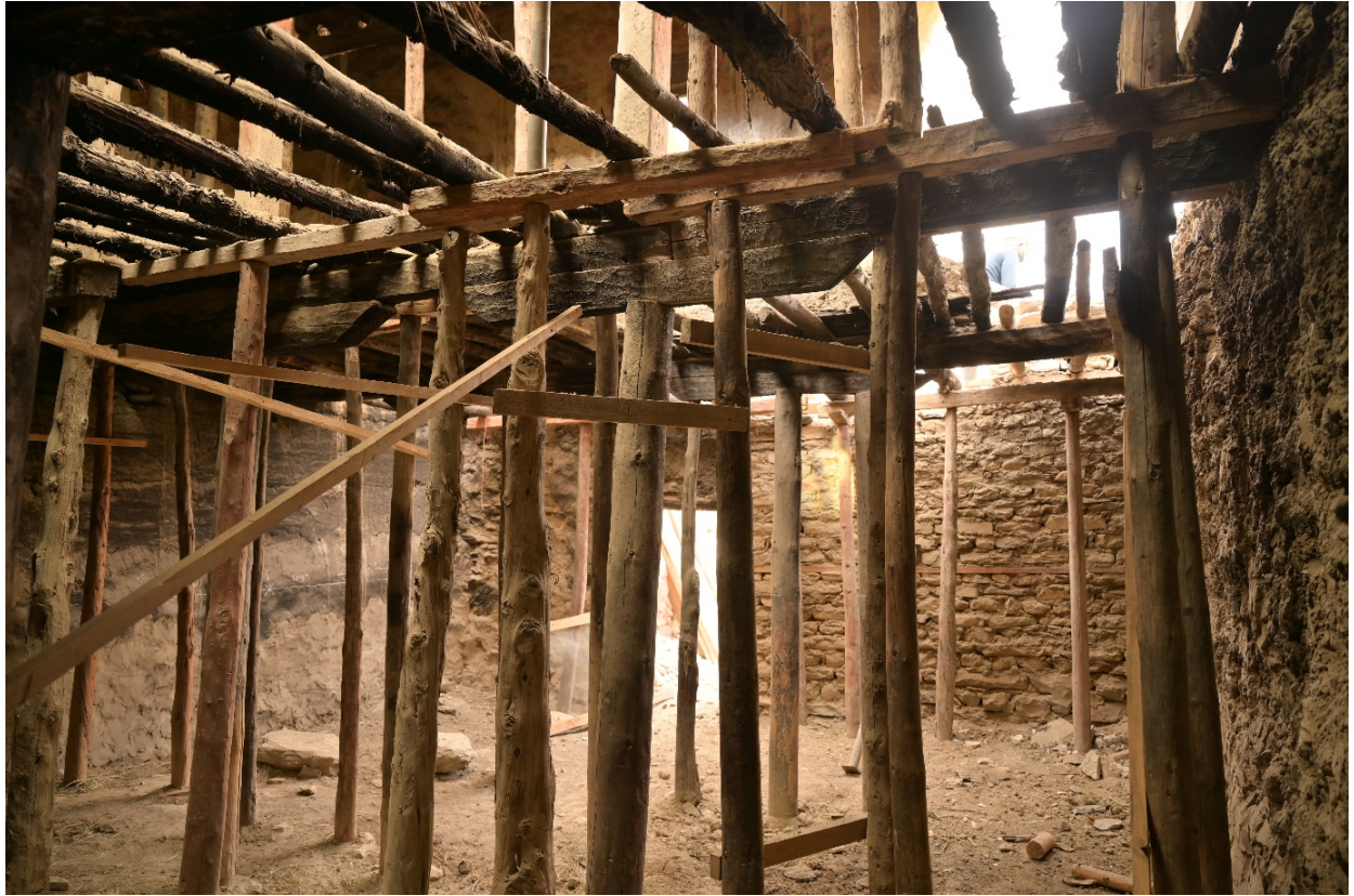
Figure 34: Installing supports for the wooden members installed before dismantling the ground floor support.
