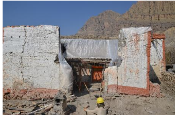
Figure 8: Once the entire interior structure was dismantled, the wall paintings were protected with tarpaulin.
