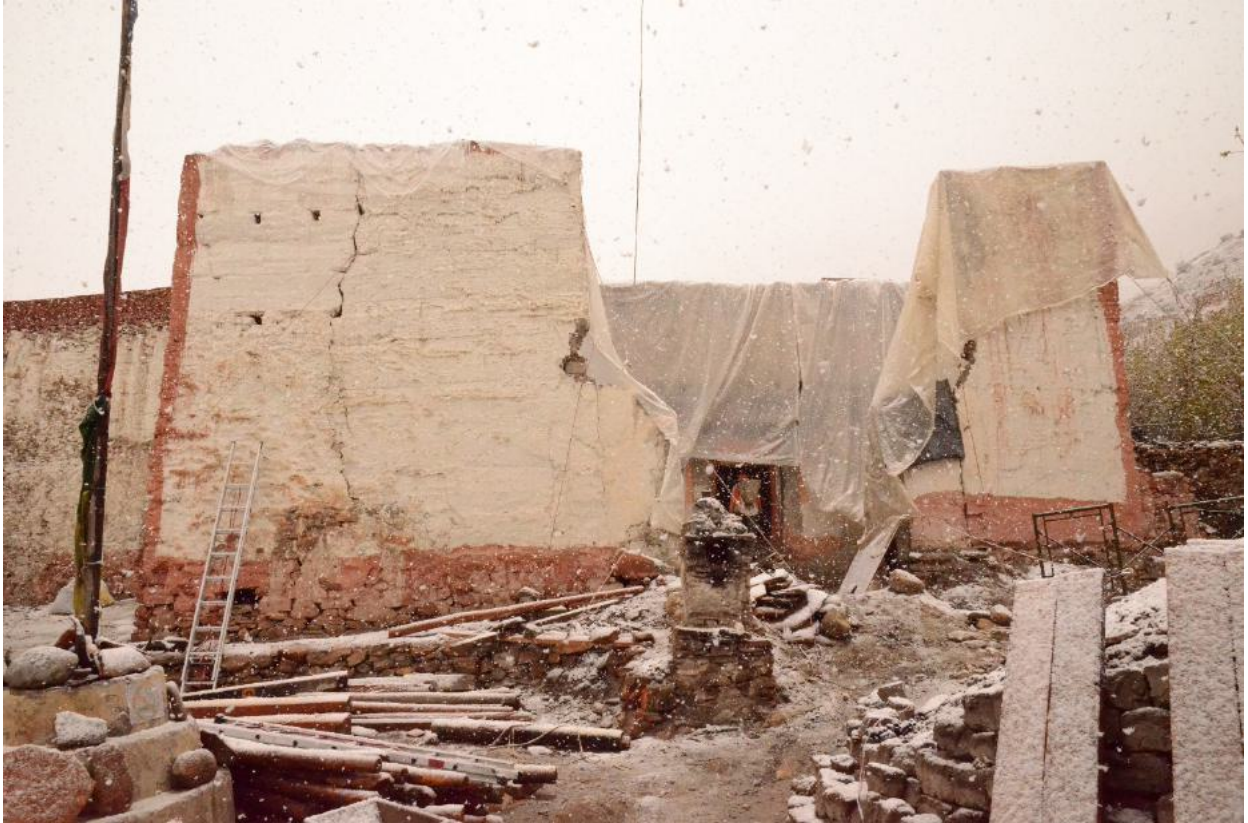
Figure 51: The entry hall with its murals covered with tarpoline to prevent damage from rain and snowfall.
