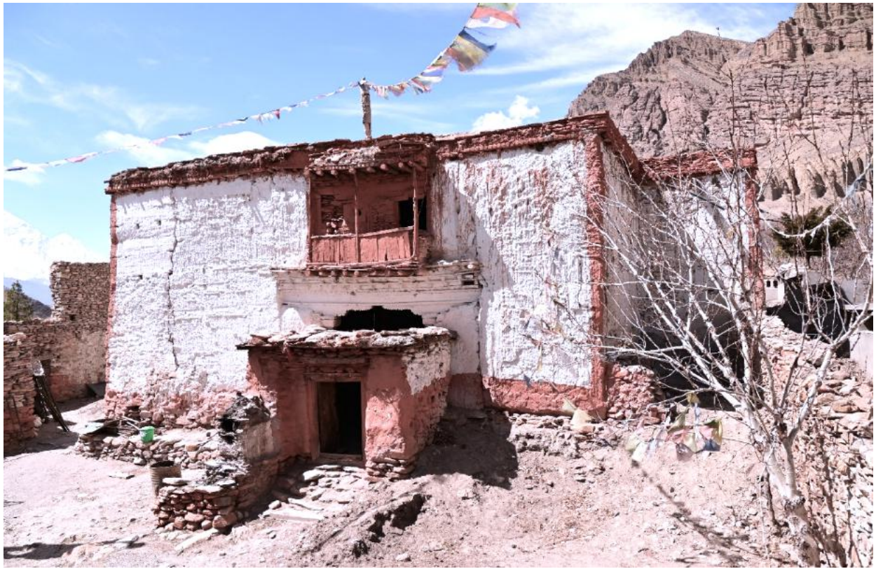
Figure 1: Photo taken before work started to dismantle the interior of the entry hall of the building.
