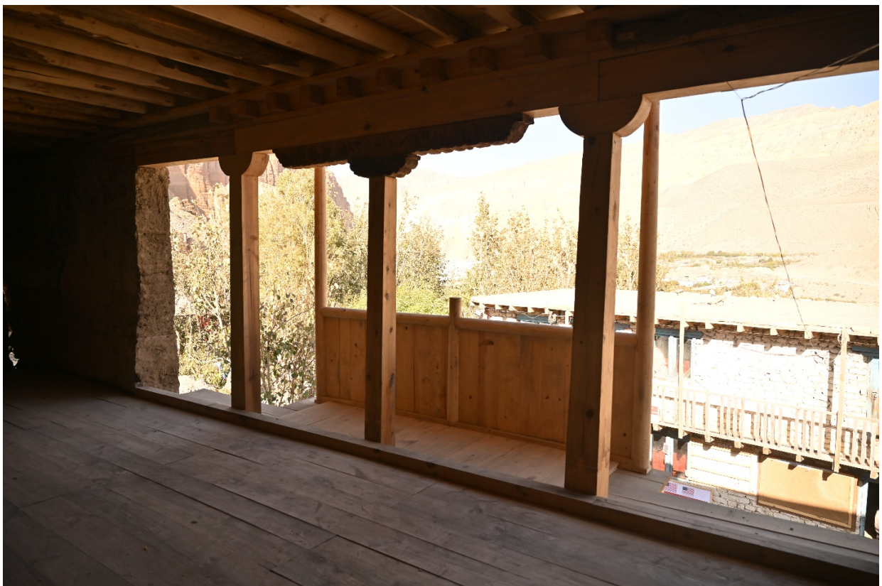
Figure 18: Photo showing the new flooring and balcony in the room above the entry to the monastery.
