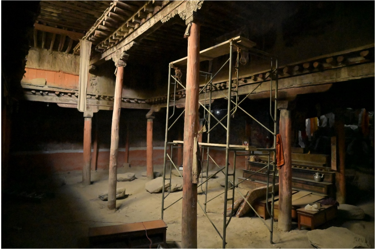
Figure 20: The scaffolding set up to be able to measure the detail of columns.
